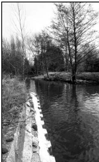
Hard revetment provides no bank side or marginal habitat.
